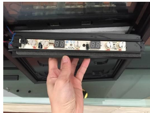
4. Pull out old temperature controller, disconnect the wire connector and replace with new controller.
